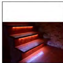
(F) UNDER STEP & HAND RAILS STRIP LIGHTS TO ILLUMINATE STEPS (T.B.D. BY ARCU)
