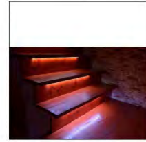
(F) UNDER STEP & HAND RAILS STRIP LIGHTS TO ILLUMINATE STEPS (T.S.D. BY ARCH)
