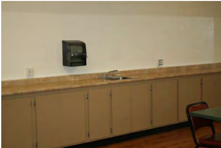
Figure 8 – Building A, non-compliant cabinet and sink
